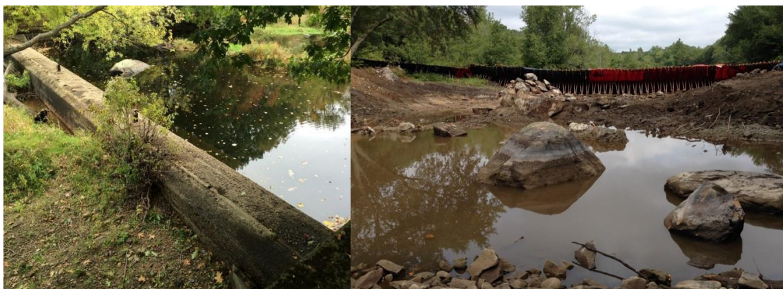
Figure C 18 – White Rock dam removal: Existing dam and accumulated sediment behind dam (left) and dam removal with upstream port-a-dam to divert flows into raceway, October 2015. Credit: NOAA Fisheries.
