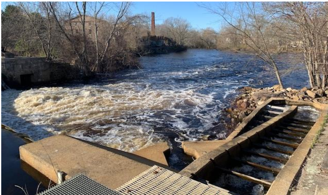
Figure C 26 - Potter Hill dam in April 2022. Narrow spillway encumbers excessive flows, creating broad hydraulic at toe of spillway. Existing fishway (circa early 1970s) functions poorly due to location of the entranceway (lower center of photo) and truncated operational flow range. The removal of the decrepit mill (background, river left) and last mainstem dam remain under consideration by the Town of Westerly and Rhode Island Superior Court in 2022. Credit: NOAA Fisheries.
