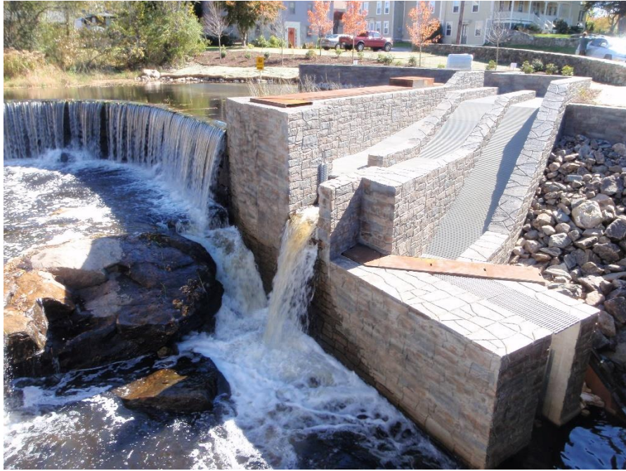
Figure C 25 – Horseshoe Falls dam with Denil fishway and eelpass, completed 2012. Credit: NOAA Fisheries.
