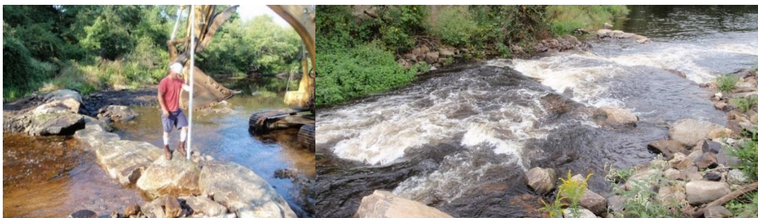
Figure C 24 – Modification of the backwatering weirs downstream of Lower Shannock Falls Dam removal to improve passage efficiency (left – 2011) and view of the backwatering weirs during low fish passage flows (right – 2012). Credit: NOAA Fisheries.
