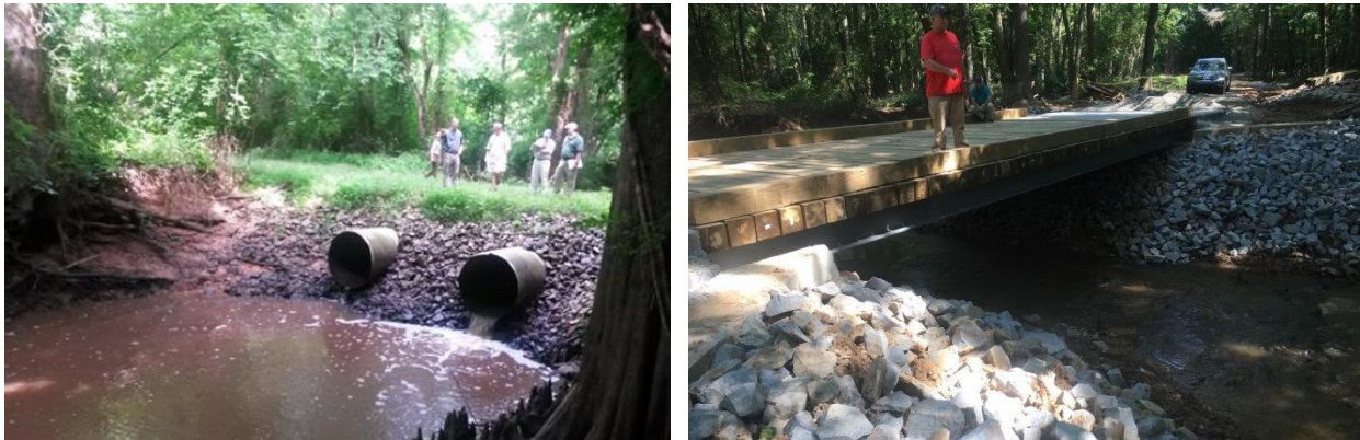
Figure C 45- Perched culverts (before) and bridge (after) at Phase 1 location on Ware's Gut at the RTRGC property. Credit: Aaron McCall/ TNC.
