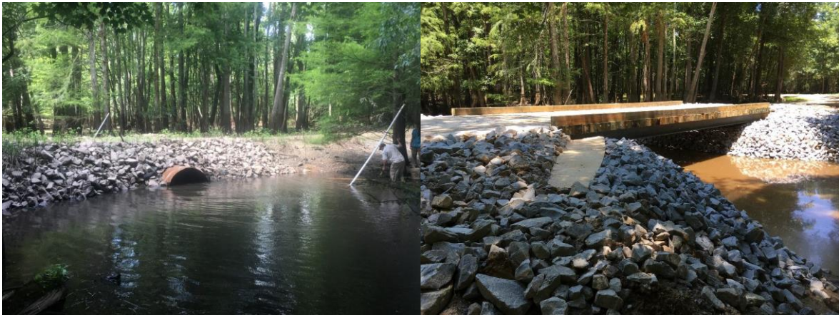
Figure C 47- Undersized culvert (before, left) and bridge (after, right) at Phase 3 location on Ware's Gut at the RTRGC property. Credit: Aaron McCall/ TNC.
