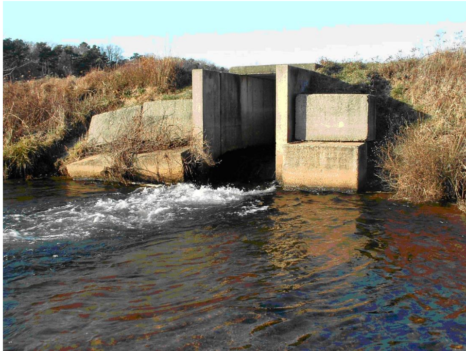
Figure C 9 – Middle Bog Dam, 2018. The Coonamessett structures were earthen dams with low-head concrete spillways and failing culverts that were effective as herring passage barriers. Credit: Town of Falmouth, MA.
