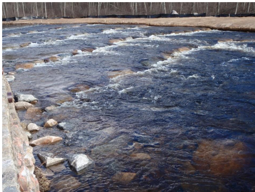
Figure C 21 – Kenyon Mill step-pool NLF, uppermost fish passage site, completed 2013. Credit: NOAA Fisheries.
