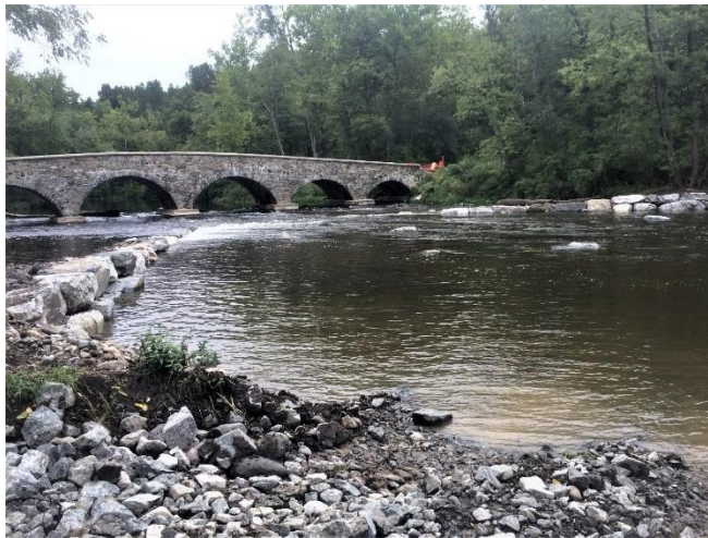
Figure C 31 - Brugler Bridge rock vane construction, view from downstream. Credit: Beth Styler Barry/ TNC.
