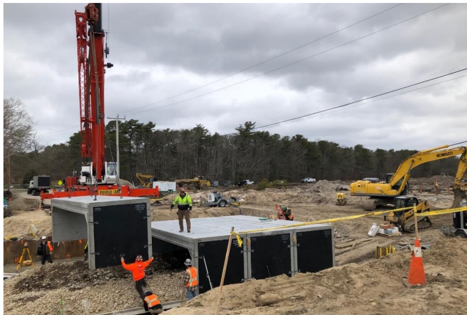
Figure C 11 – New, fish passage-friendly culvert installation at John Parker Road, May 2020. Credit: NOAA Fisheries.
