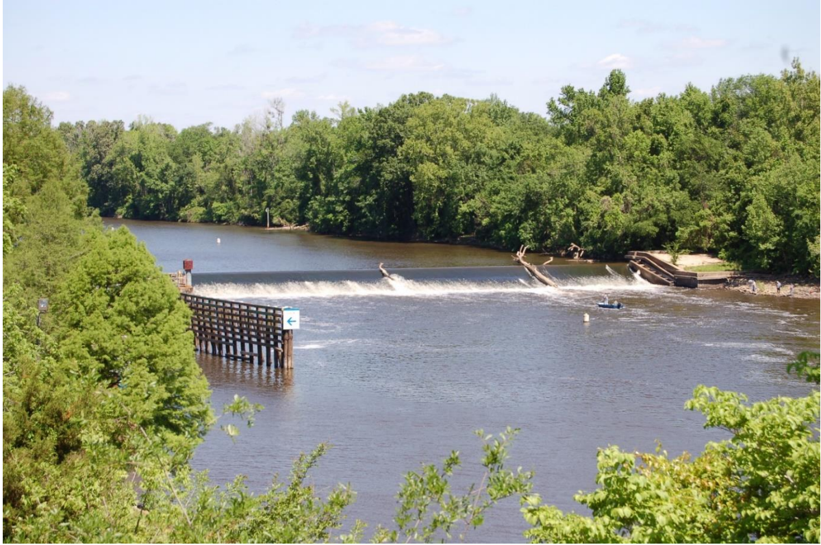
Figure C 49 – Original Lock and Dam No. 1 on the Cape Fear River, NC. Credit: NOAA Fisheries.
